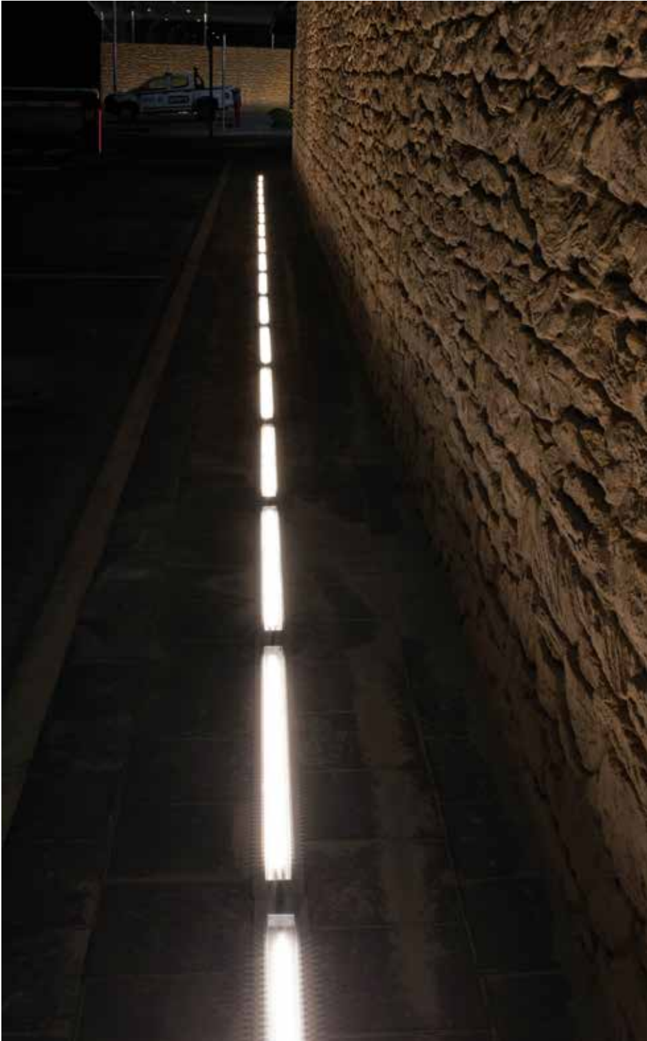
Highlighting the outer wall's stone work, LED Linear's Kalypso HYDRA HD15 linear LEDs add a decorative touch to the industrial location.
